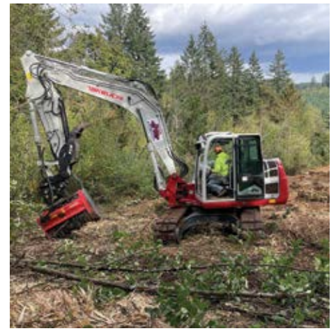
About one acre of ice damaged alder was masticated by American Onsite in preparation for replanting. PHOTO BY GLENN AHRENS
