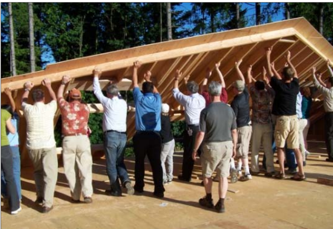
Chamber members' of Oregon City, North Clackamas County and West Linn push up south wall of the new classroom.
